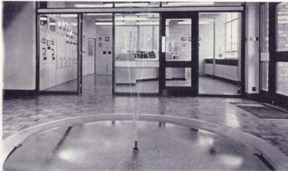
Entrance Hall, Sluval Treatment Works
